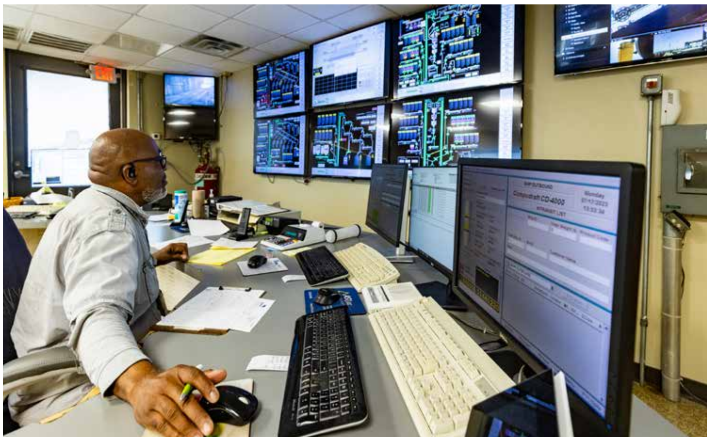
Control Room Operator Linel Wrice monitors ship-loading activities at the TEMCO export terminal in Houston, Texas.
